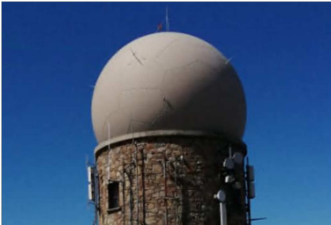
Figure 10. Dooncarton - Secondary Surveillance Radar (SSR)
